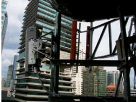
By deploying their access point on an existing water tower, Maxis leverages light infrastructure and flexible deployment options in Malaysia.
